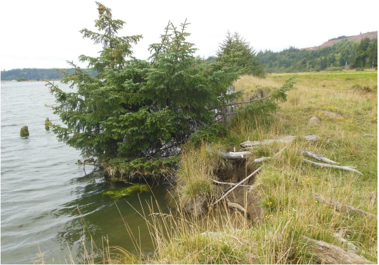
13. Typical eroded section of river bank
