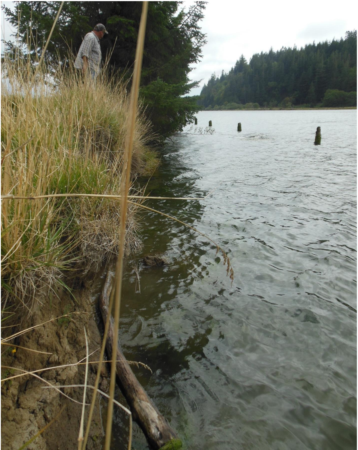
12. Undercut banks where spruce are toppling due to being planted too close to river historically.
