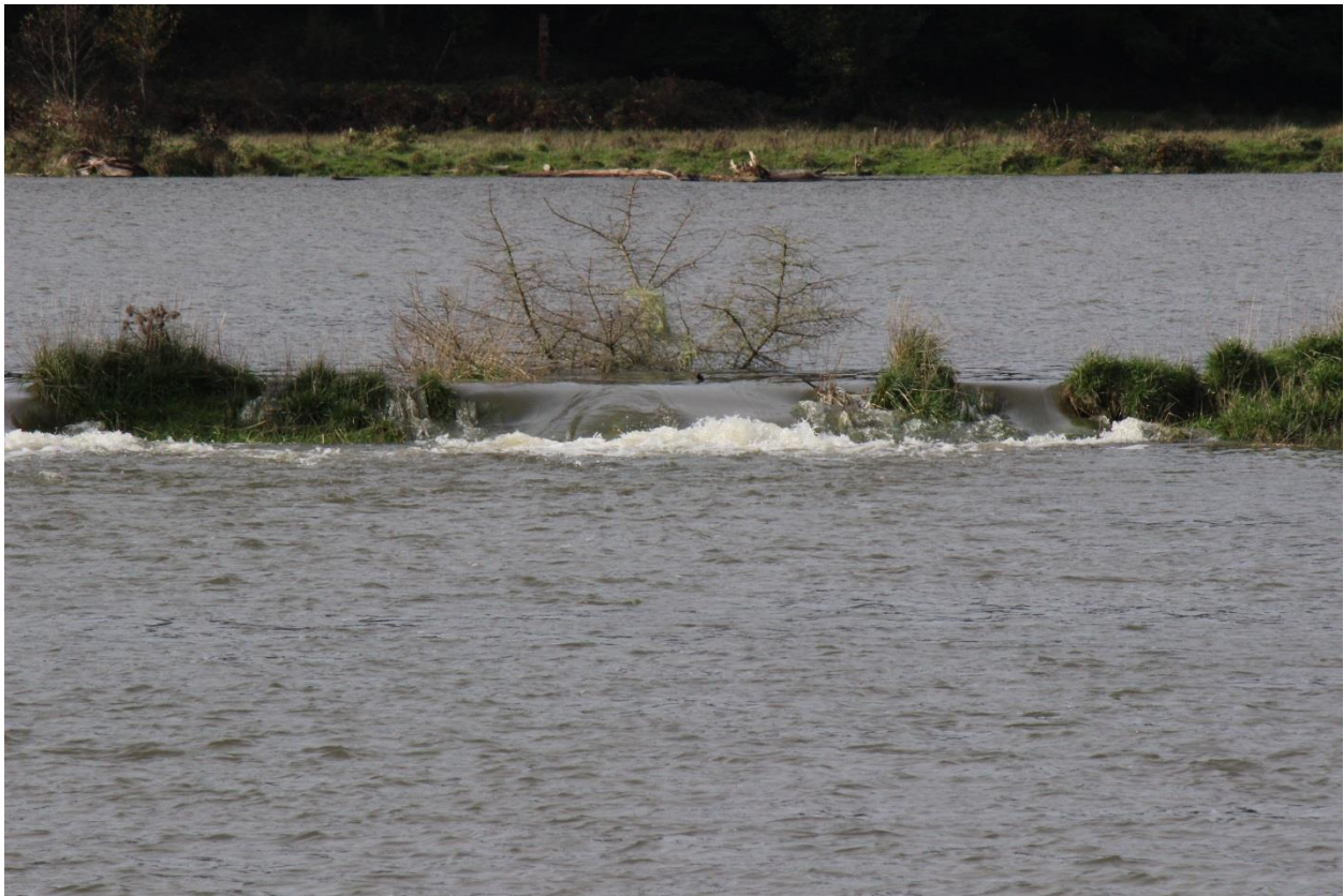
5. Breached section of dike on project area that has failed; photographed during winter high tide/ storm surge
