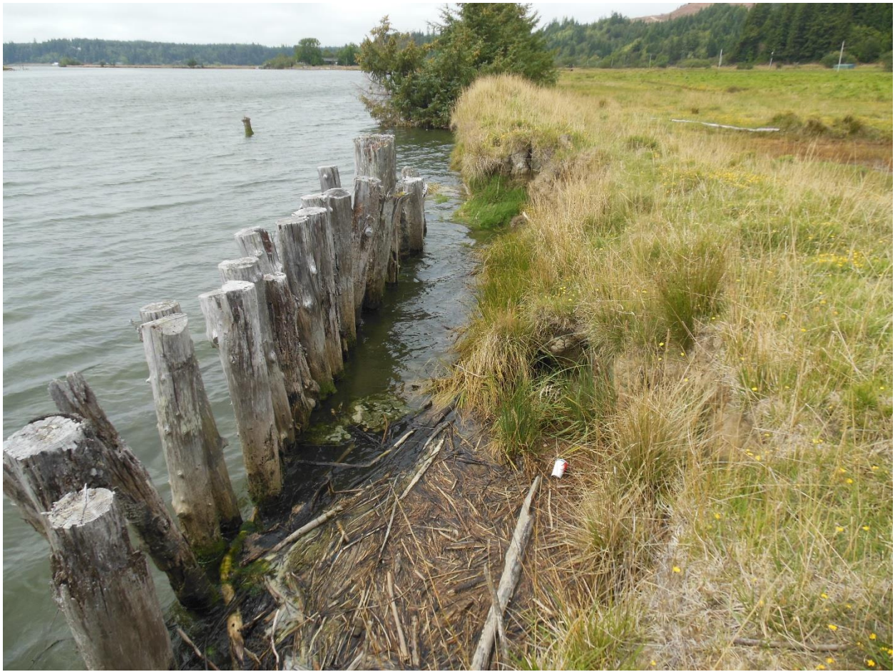
14. Evidence of past efforts to protect and reinforce the dike; pilings originally placed at toe of dike. River has eroded toe of dike due to poor placement.
